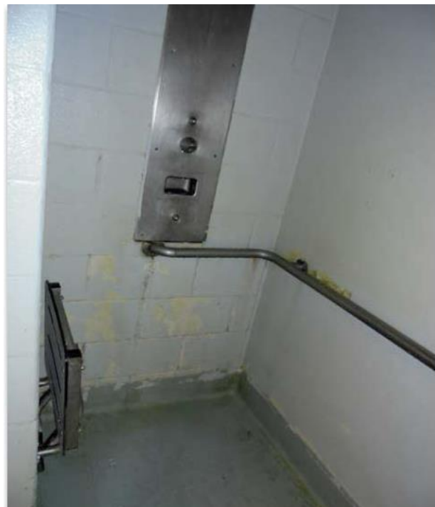
A shower stall at Adelanto Detention Center in May 2018 (Credit: DHS Inspector General )
